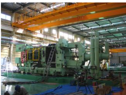
DC machine moved from Hamamatsu to the third casting plant at Tokai Plant
